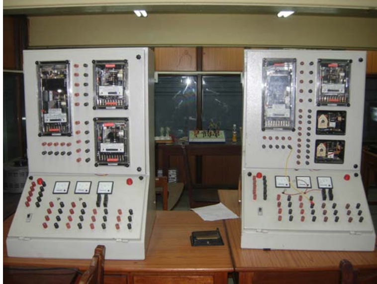
Induction and static relays on panels
